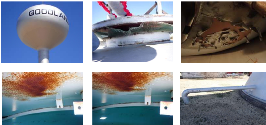
Pictures of Power Plant Tank - Cone-top by Power Plant - The top priority should be working on the roof. Many of the clips holding the roof down are broken. The gap at these clips really needs to be addressed. Water Tower roof "shall be watertight with no openings except properly constructed vents, manways, overflows, etc."
